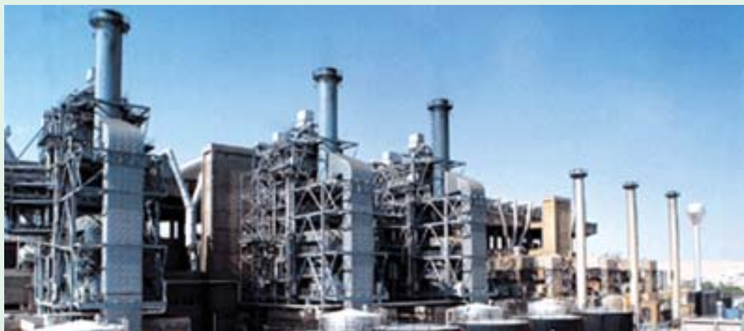
An overview of a thermal power plant
